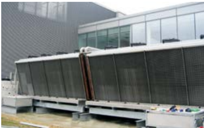
Mountair Datacenter Cooling, PGS London
